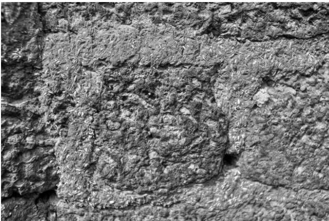
Fig. 9: Ancient laterite brick wall, linked by a mixture of young mud - rice husk
