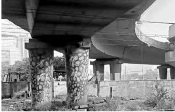
Fig. 2. Columns of the flyover at A busy elevated road junction in Turbhe, Navi Mumbai exterior paint. 2021
