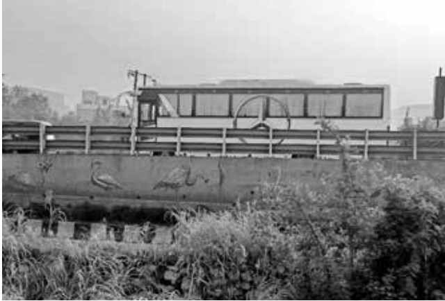
Fig. 4. Side wall of a flyover enroute Koparkhairane, Navi Mumbai. exterior paint. 2019
